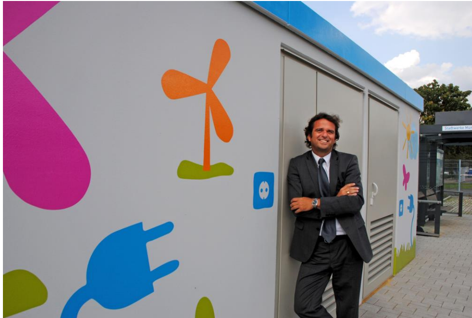
Fast Charging Station Münster
